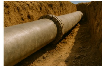
Large Water Pipes ( \geq 800\text{mm} diameter)
