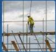
Unsafe Working at Height
