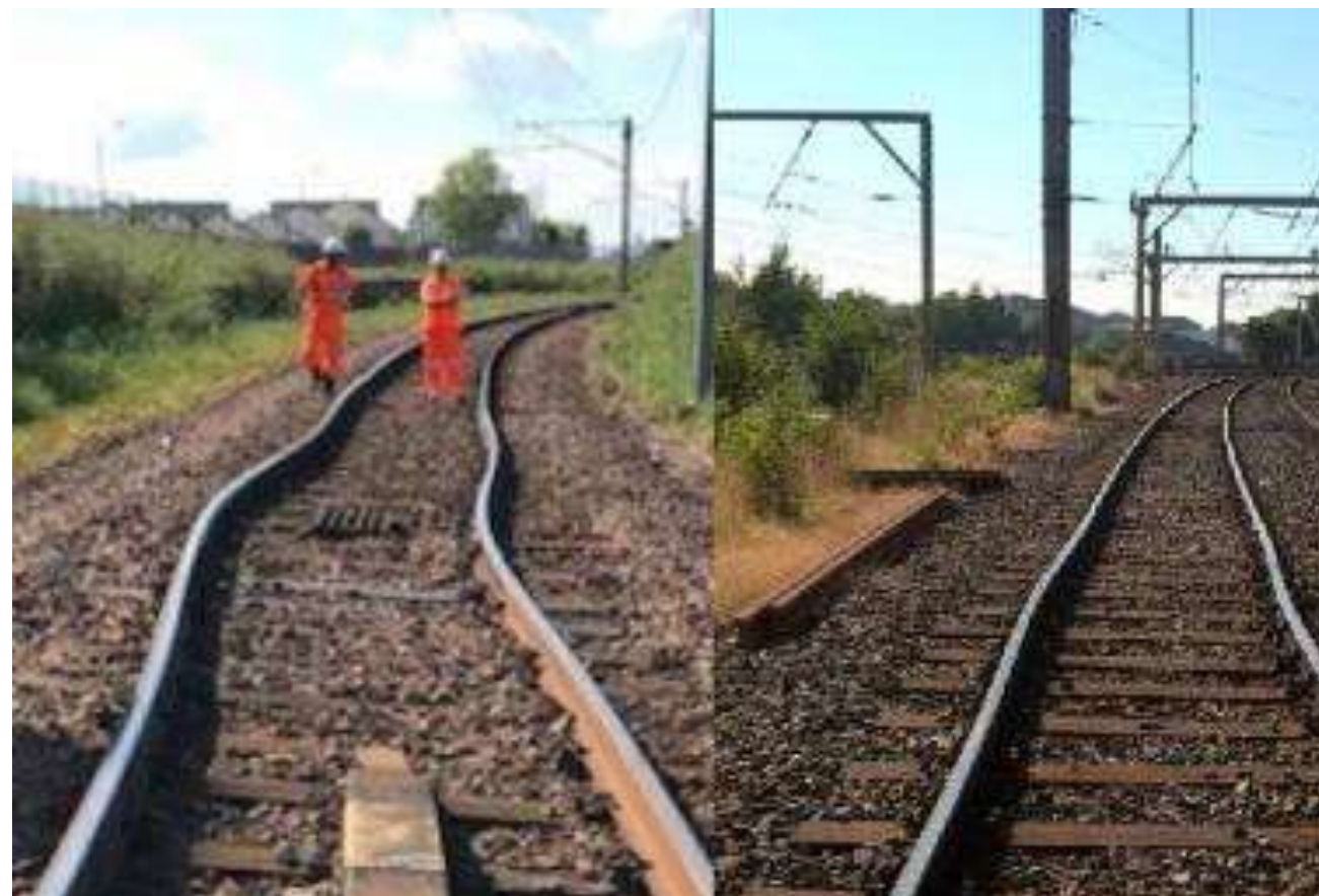
Buckled railway tracks in UK during heatwaves in July 2022
